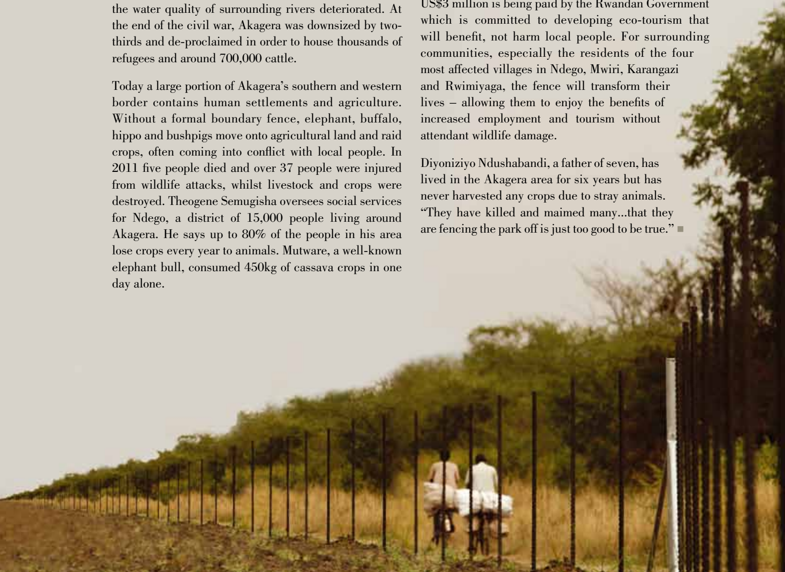
Construction commenced at the end of the year on the western boundary fence – Sarah Hall
